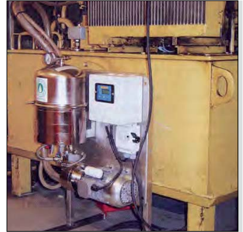
The 1300ltrs. oilreservoir, here shown with a Europafilter cleaner assembled. The filter cleans in a kidney loop.
